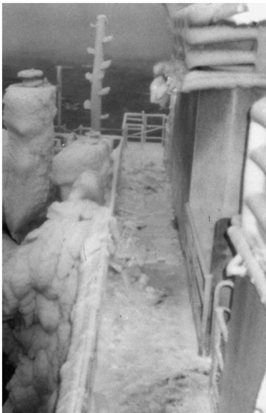
Fig. 6. Iced air vent on right, and ice littering deck of semisubmersible platform Ocean Bounty (Courtesy U.S. Minerals Management Service).
